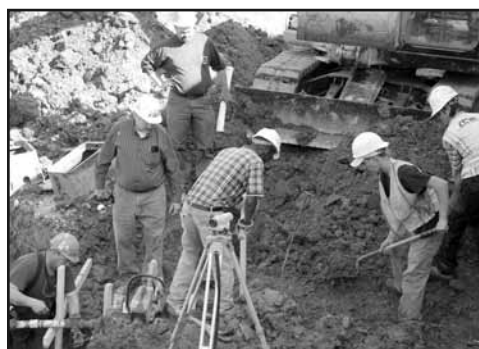
Workers dig trenches to put in new waterlines for the pool and spa
