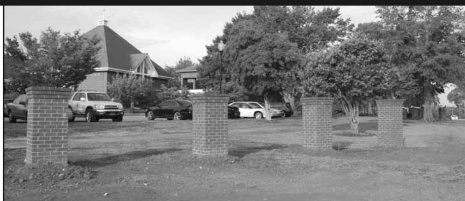
Newly built brick piers dry in preparation for the installation of new signage along Highway 76
